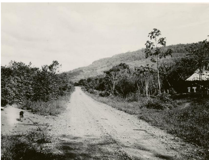
At Rio Madronal - looking toward David. The road having a badly worn gravel surface. 17 March 1942
